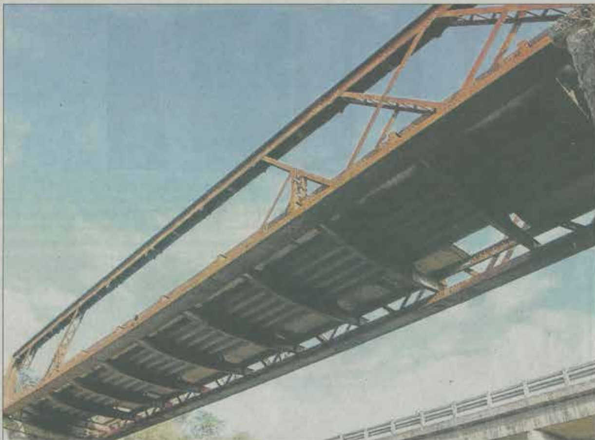
FALLING DOWN: This photograph shows how thieves are stripping the Kwelera Bridge of iron to sell as scrap metal
